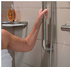
Riser safety grab bar
